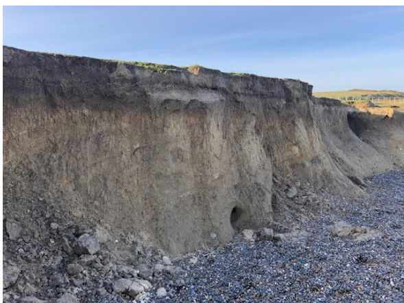
Fig 3.4E. Cliff face condition.
