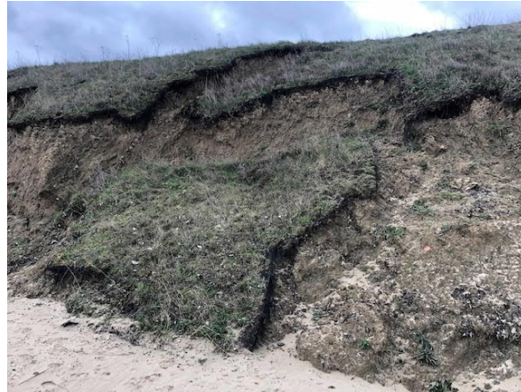
Fig 3.1E. Cliff condition at beach level.
