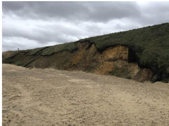
Fig 3.1D. Cliff condition at beach level.
