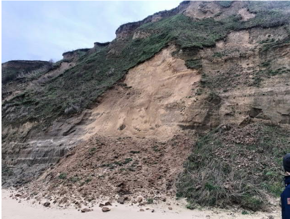
Fig 3.2E. Cliff condition at beach level.
