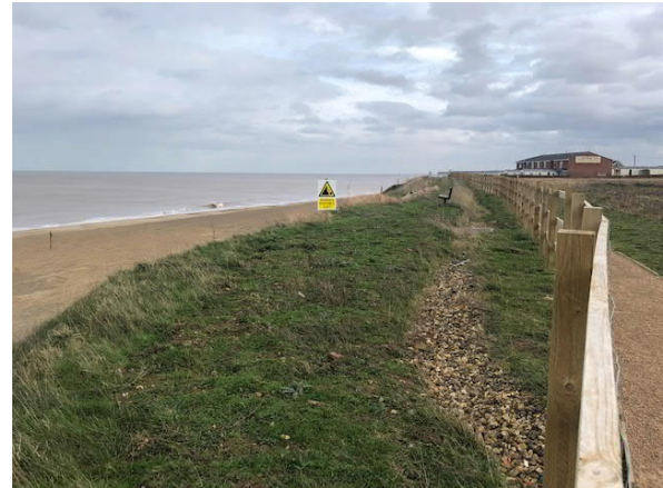
Fig 3.1B. Embankment fenced off due to erosion.
