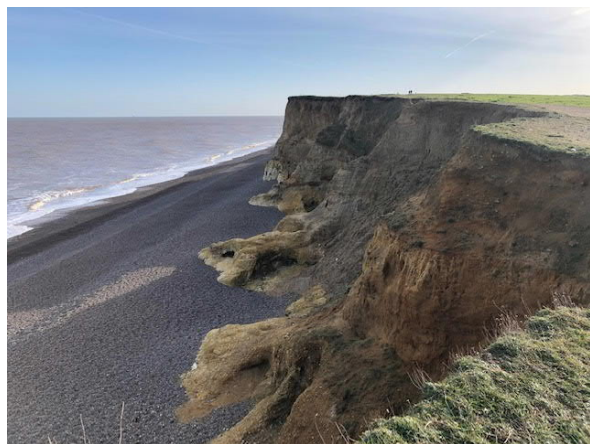
Fig 3.3D. Cliff face condition from top of cliff.
